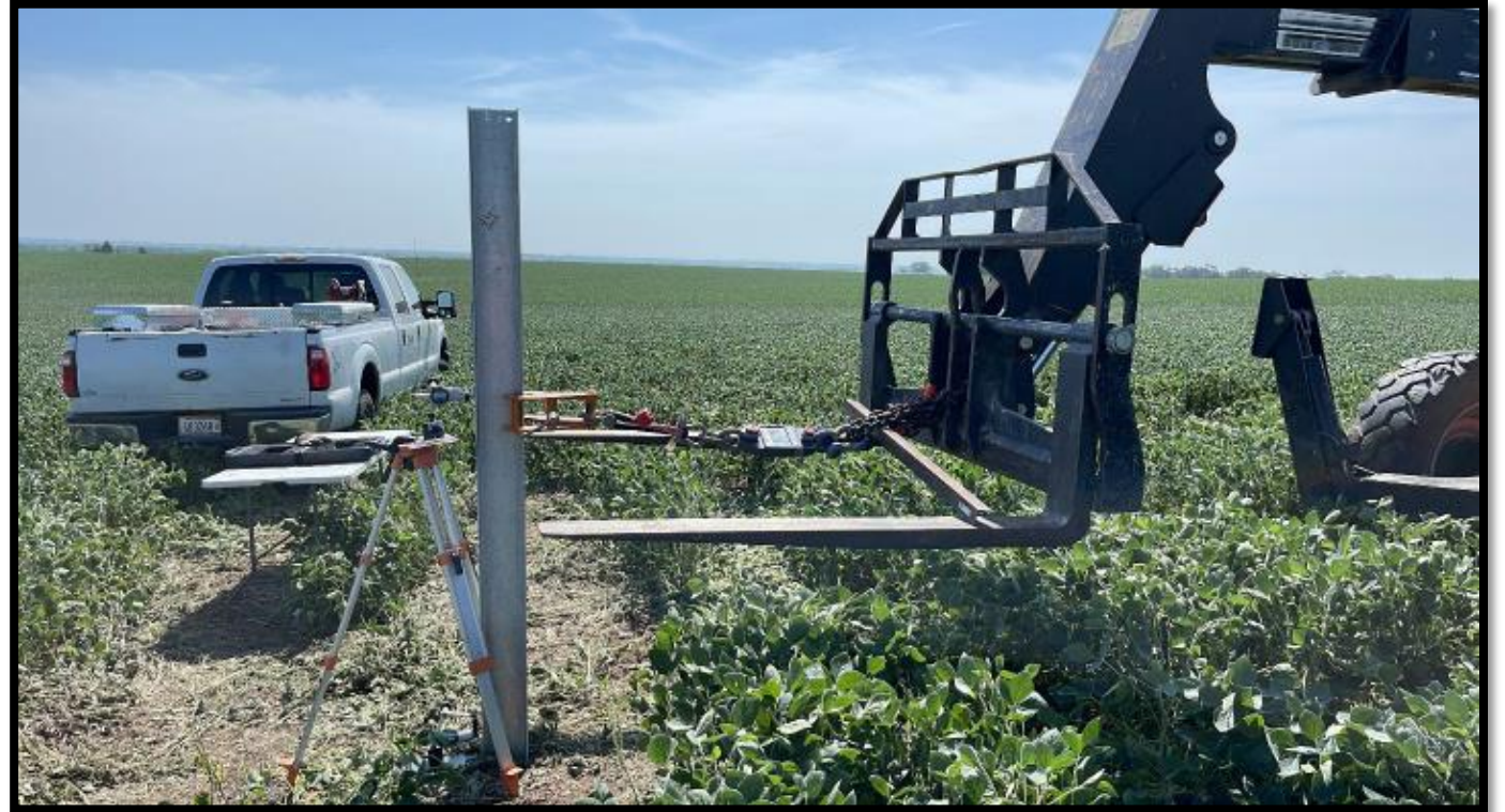
Photos of pile load test conducted at Platteview site. Testing was planned and coordinated with landowners.
