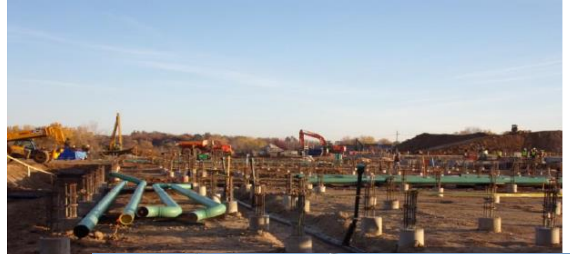
Auxiliary Cooling & Waste Disposal Lines for Engine Hall 1
