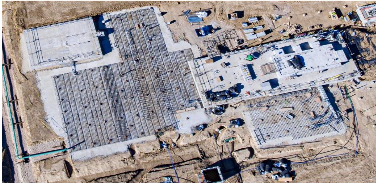
Unit #1 Generator/Gas Turbine at TCS site
