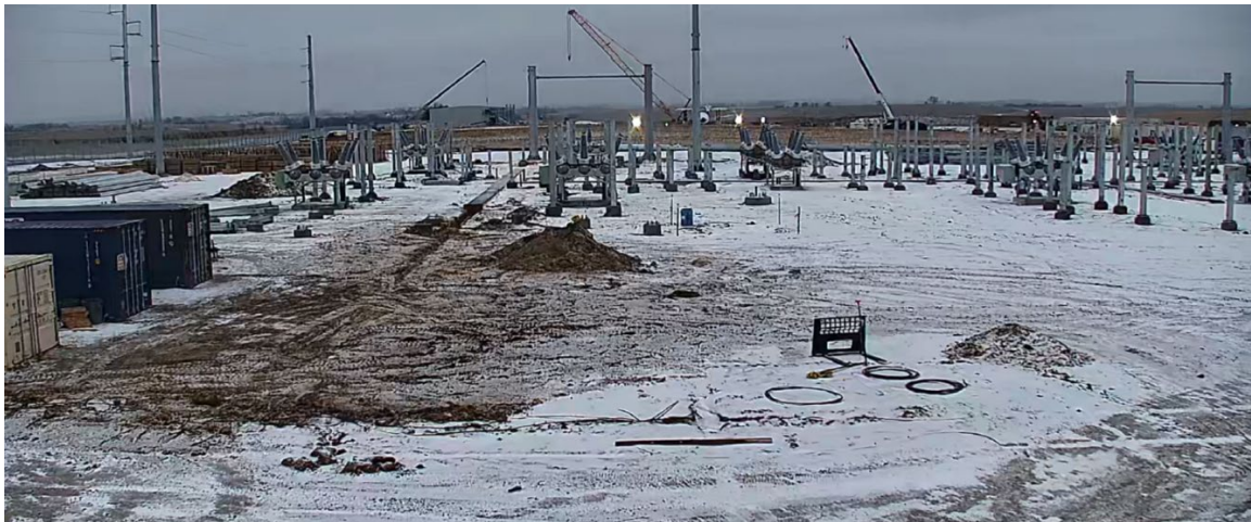
Facing South – Substation
