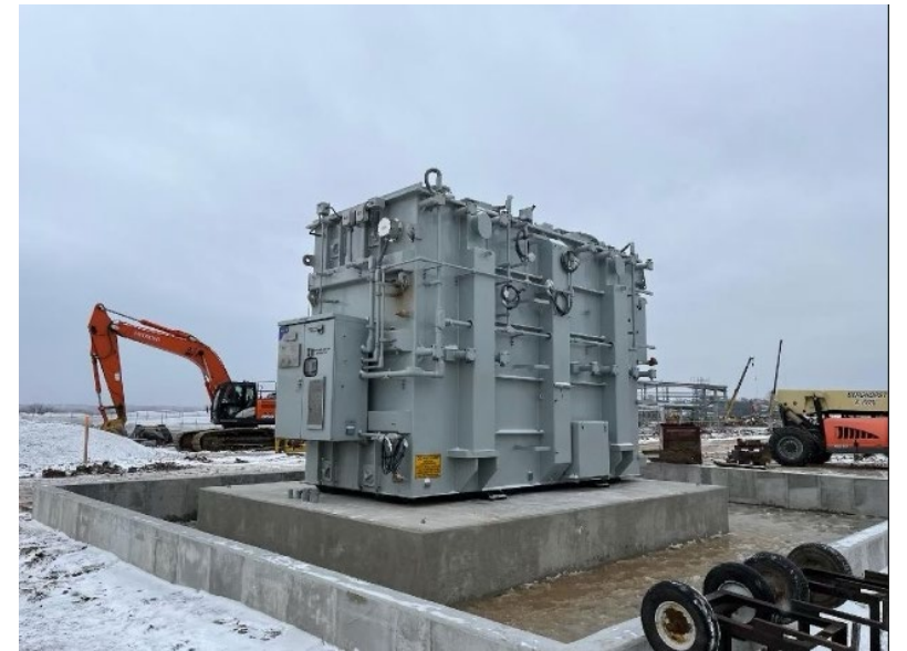
Generator Step-Up Transformer on foundation Information as of January 5, 2023
