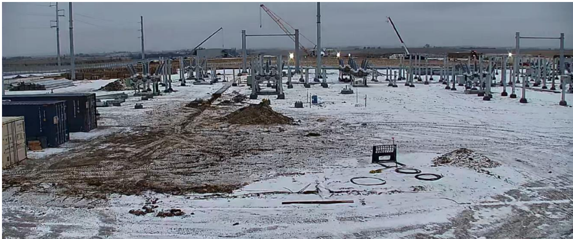
Facing South – Substation
