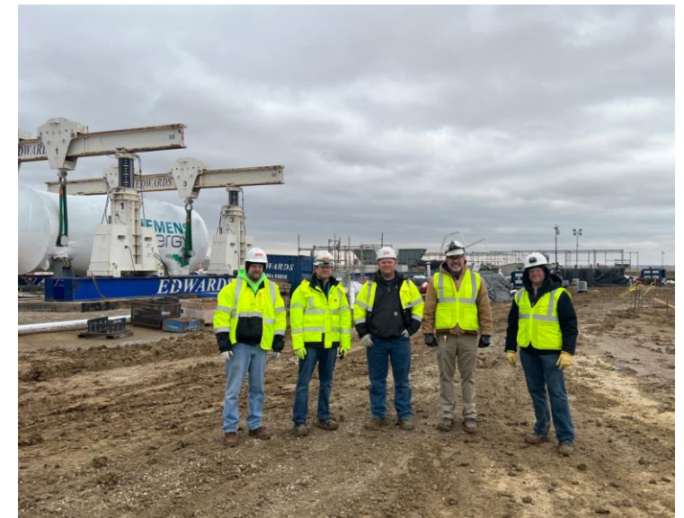
Gas Turbine #1, OPPD Staff Observance
