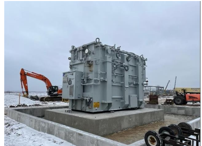
Generator Step-Up Transformer on foundation Information as of January 5, 2023
