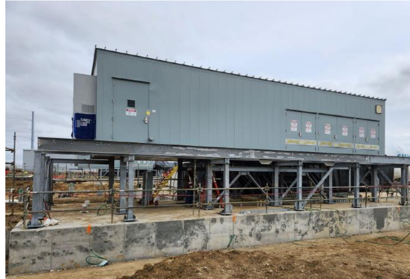
Unit #2 Electrical Package
