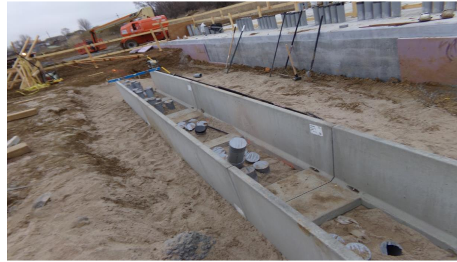
Facing Northeast – Substation Control House Duct Bank
