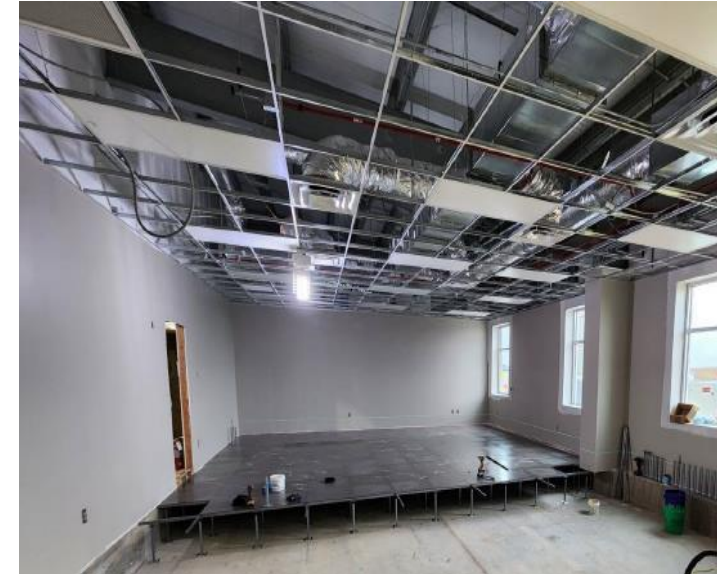
Admin Bldg. – Control Room Raised Floor
