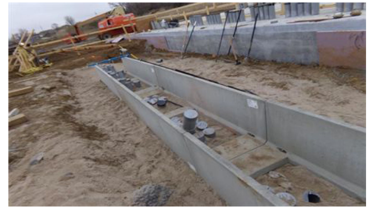
Facing Northeast – Substation Control House Duct Bank
