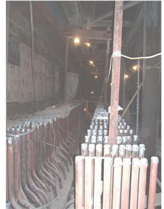
Reheater Header with Tube Assemblies
