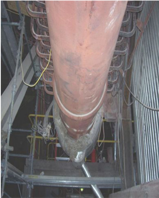
Reheater Outlet Header
