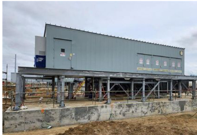
Unit #2 Electrical Package
