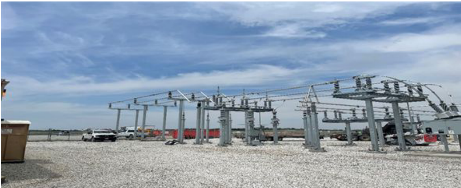
OPPD Substation – Bus Extension to AES Collector Substation
