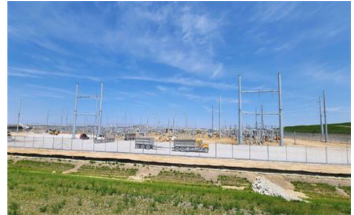
Facing North - Substation
