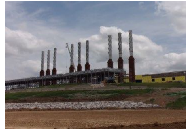
Facing Northeast – Radiators & Stacks
