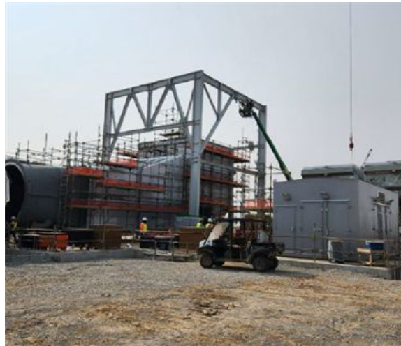
Facing Southeast - Unit #1 Stack
