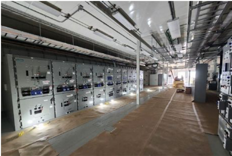
Interior of Power Distribution Center
