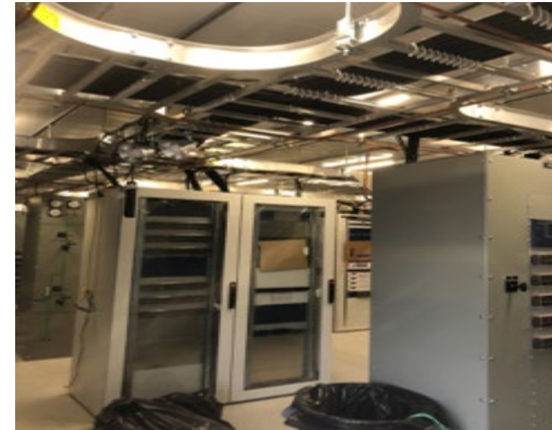
Substation Control House Wire Termination
