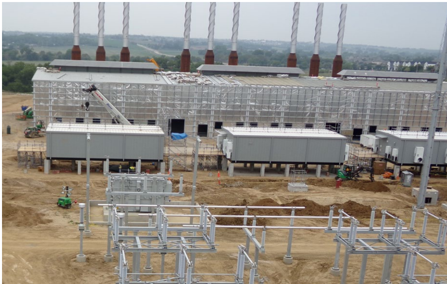
Facing West – Power Distribution Centers
