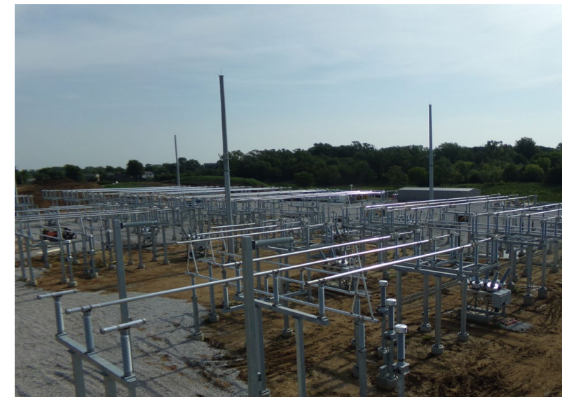
Facing Northeast – Substation
