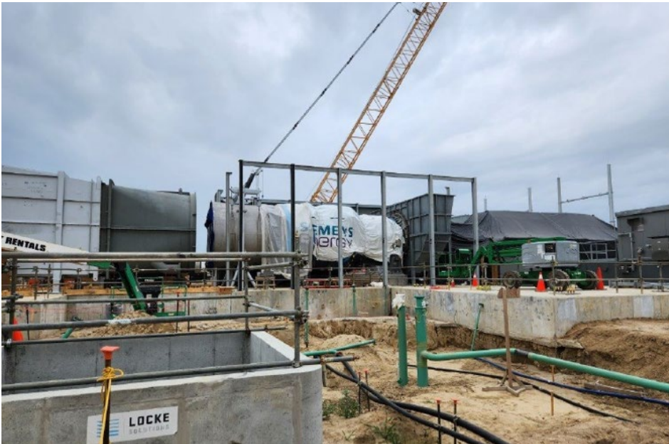
Facing Northwest – Unit #1 Turbine Enclosure
