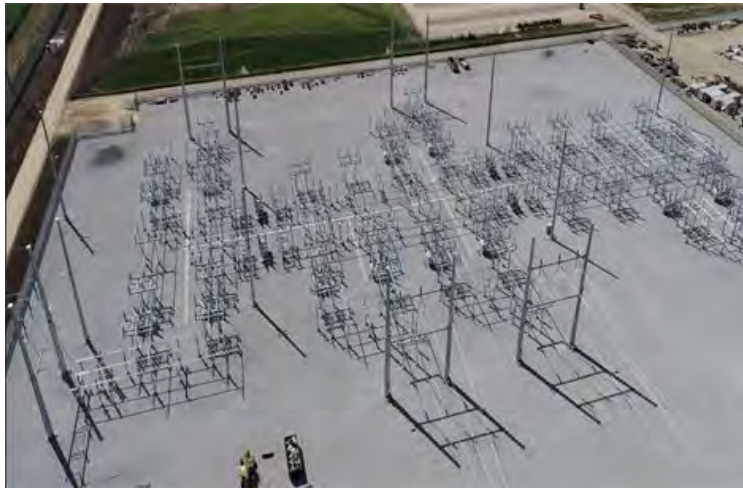
Facing South – Substation Aerial
