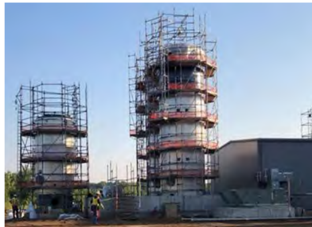
Facing North - Service Water/Urea Tanks Insulation
