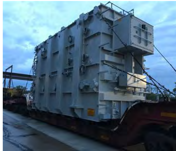
Generator Step-Up Transformer
