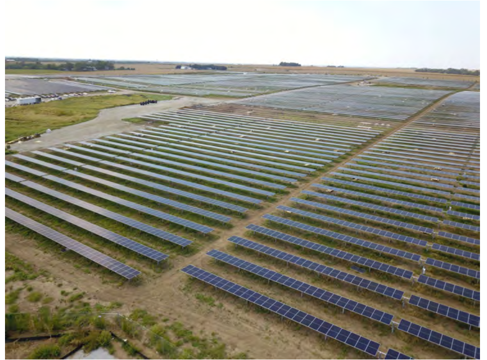
Platteview Solar – Aerial of Central Parcel
