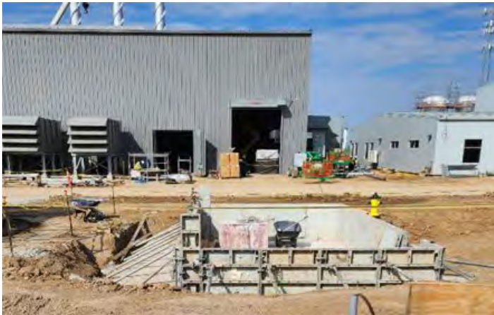
Facing West - Emergency Diesel Generator Foundation
