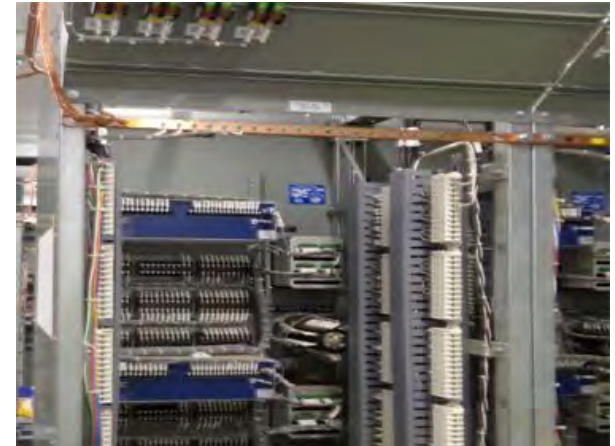
Substation Control House
