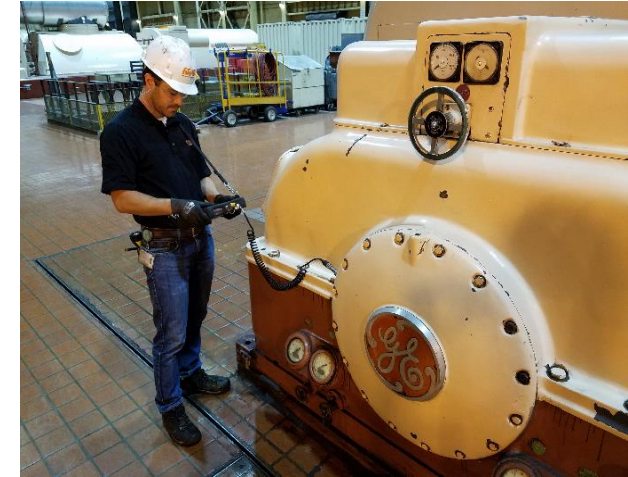
Engineer monitors vibrations on a generator exciter at North Omaha
