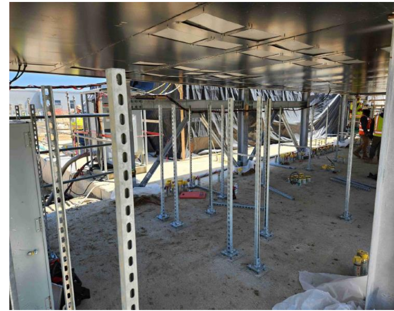
Unistrut for Cable Tray – Electrical Package
