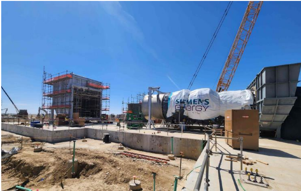
Facing West – Unit #1 Inlet, Turbine, Exhaust, & Stack
