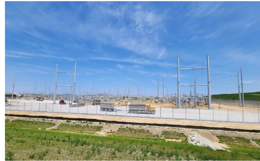
Facing North - Substation
