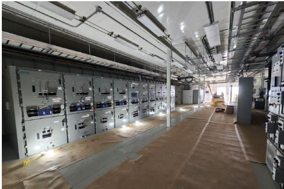
Interior of Power Distribution Center
