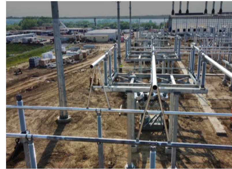
Facing West – Substation: Bus Installation
