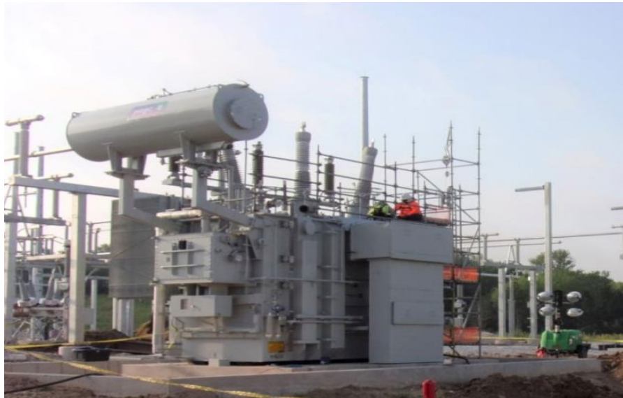
Facing Southeast - Generator Step-Up Transformer
