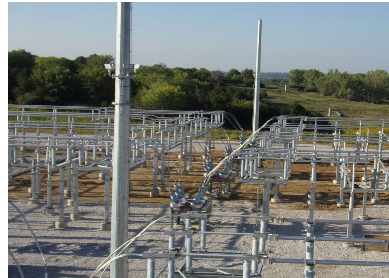
Facing South - Substation
