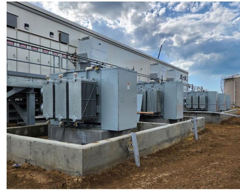
Station Service Transformers on Foundation
