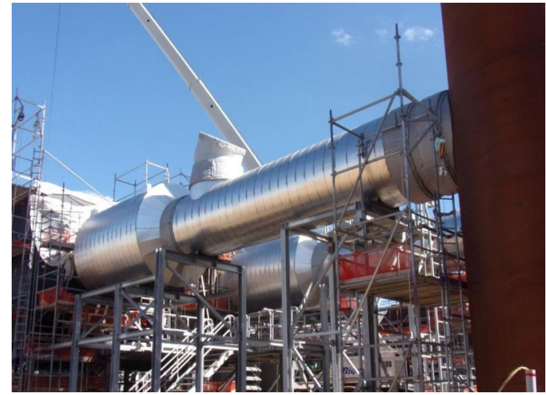
Engine Horizontal Ductwork/Insulation to Stack
