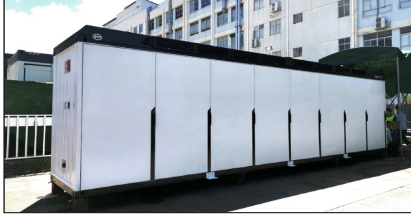
OPPD's battery container will look similar to this.
