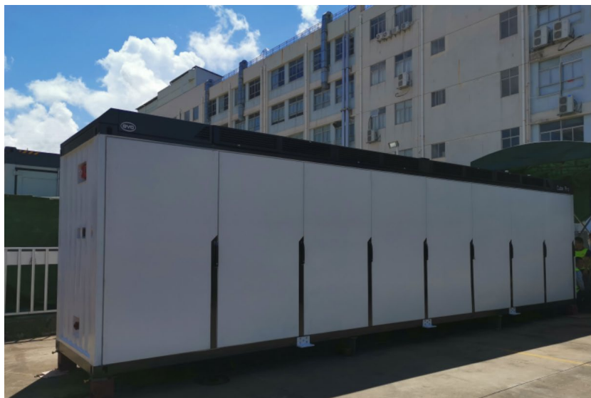
Figure 5-83 Representative Project for BRIGHT (Photo credit BYD)
