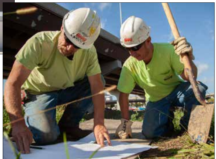
Paul Latoza, construction working crew leader, left, and Matt Liston, underground helper, review plans for a new underground vault to serve downtown Omaha.
