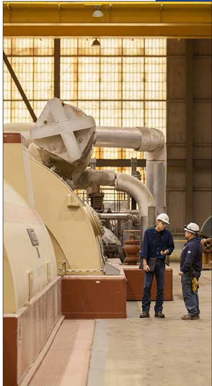
Ryan Gerdts, manager of Station Operations at Nebraska City Station, left, talks with Equipment Operator George Schworm near the turbine.
