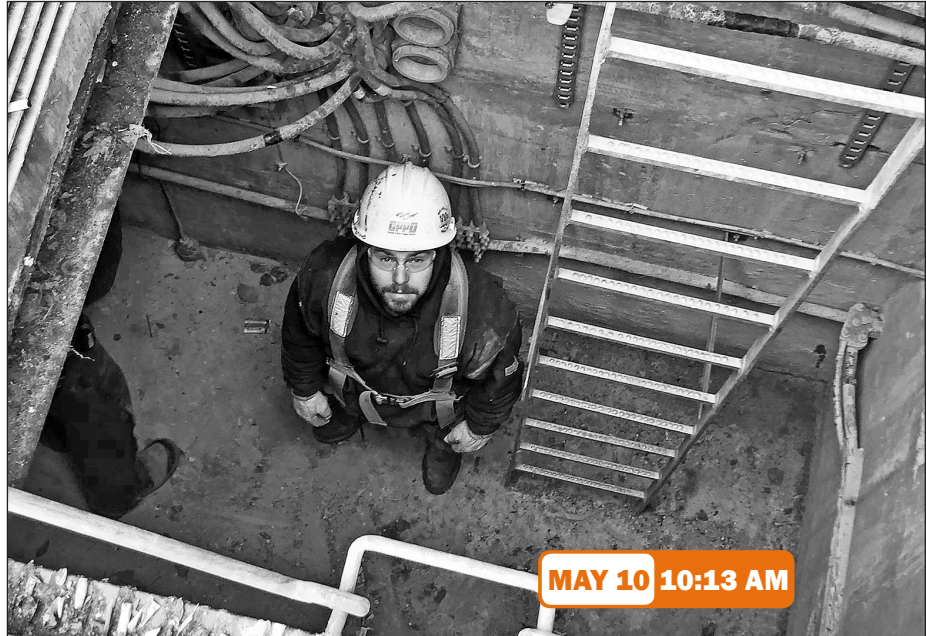
Wyatt Story, an apprentice cable splicer, works in a downtown Omaha vault.
