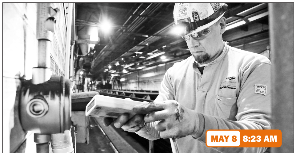
Wade Hatzenbuehler, combustion turbine technician, is among the many trades people, such as electricians, welders and steamfitters, who constantly monitor power equipment.
