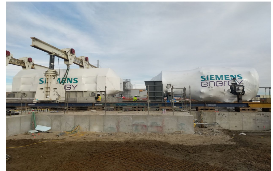
Siemens Gas Turbine/Generator Set on Foundation
