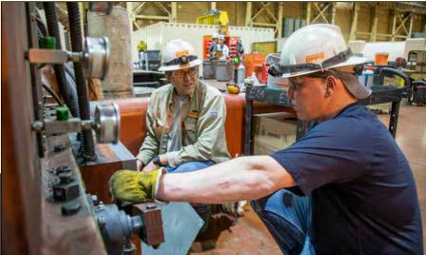
Chris Golden, left, and Tanner Lech are shown doing some maintenance work at North Omaha Station.
