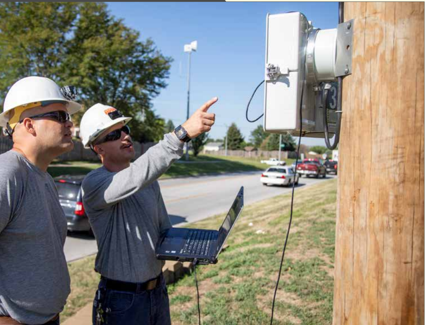
Automation Technicians Jon Willey, left, and Chad Boyce check a recloser on a pole.
