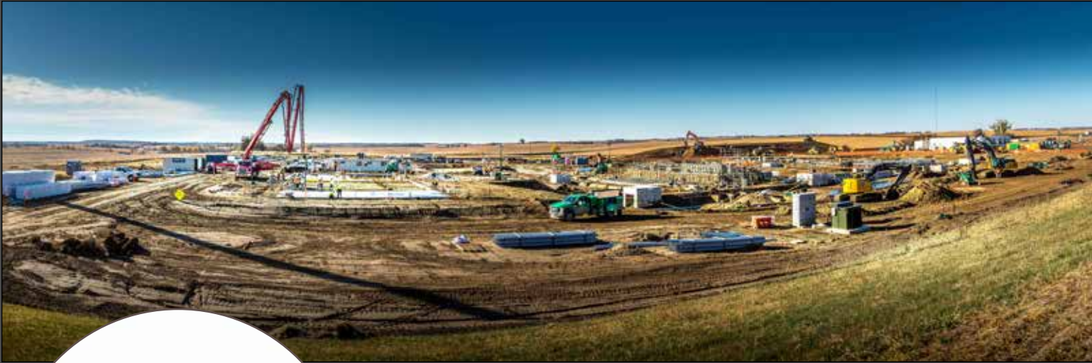
Construction is progressing at OPPD’s Turtle Creek Station, one of two natural gas plants being built.
