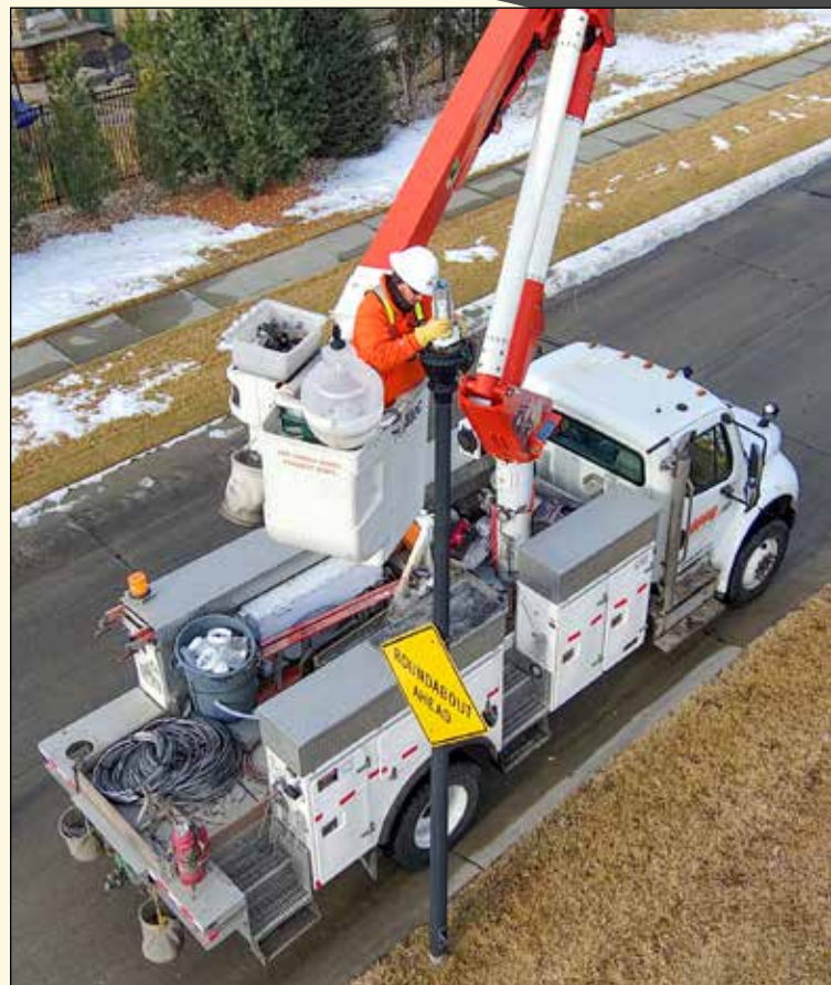
OPPD has replaced more than 90,000 streetlights with LED lights across the service territory over the past four years.
