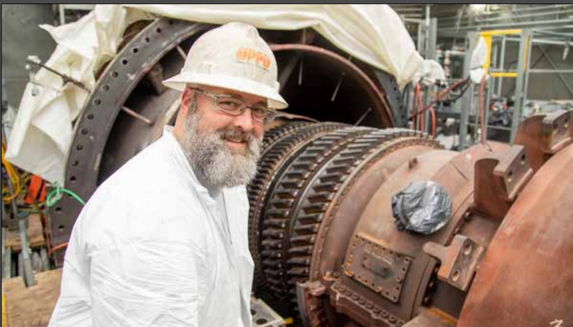
Josh Lemay, a first class machinist at OPPD, is shown checking the fit of turbine blades in front of the exhaust section at Cass County Station's unit 2. Cass County is one of OPPD's balancing stations, also known as peaking stations.
