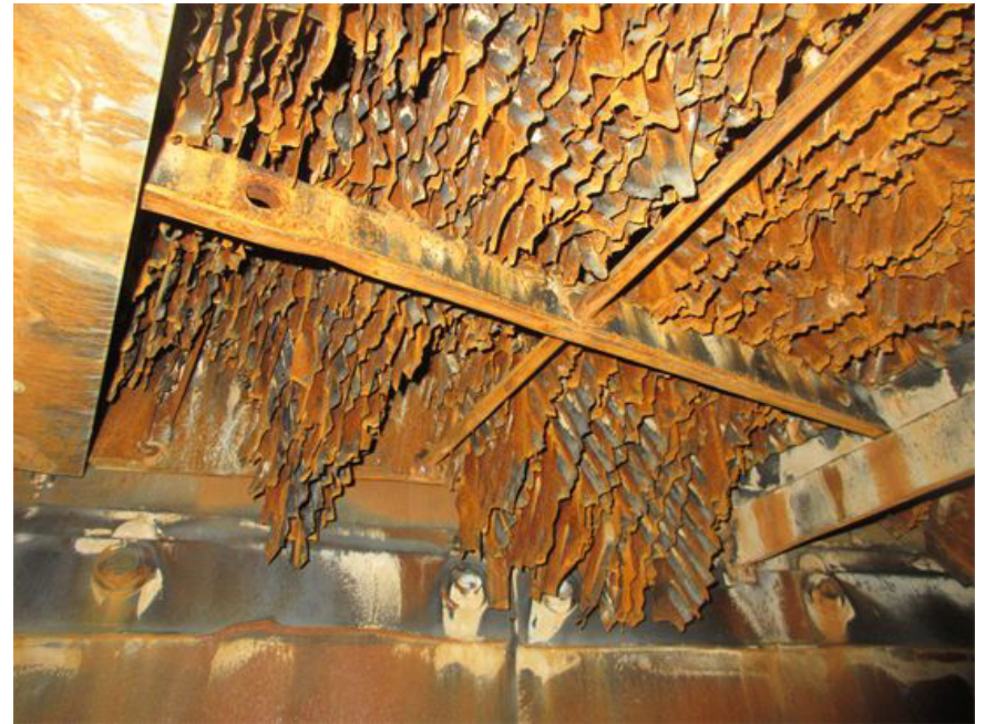
North Omaha Station Unit 4 Air heater baskets 2022
