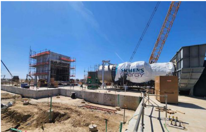
Facing West - Unit #1 Inlet, Turbine, Exhaust, & Stack
