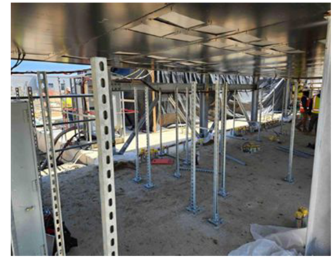
Unistrut for Cable Tray - Electrical Package
