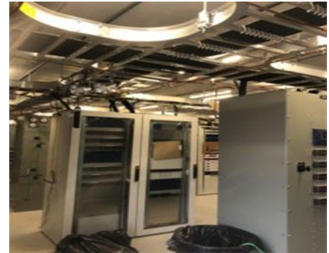
Substation Control House Wire Termination
