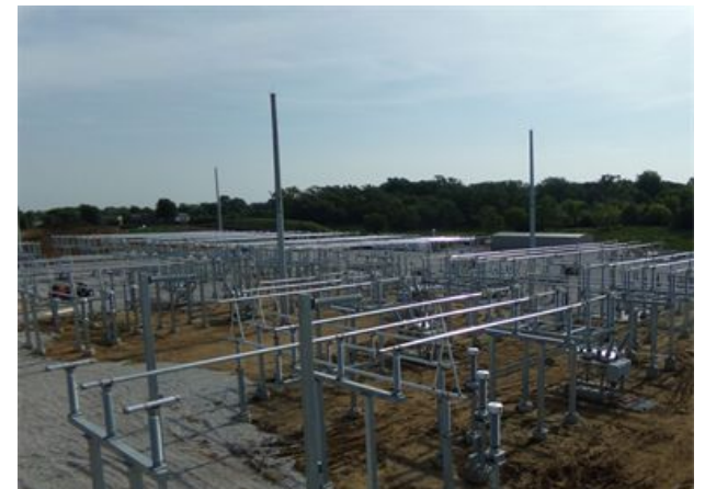
Facing Northeast – Substation
