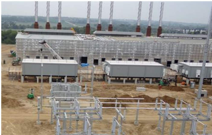
Facing West – Power Distribution Centers
