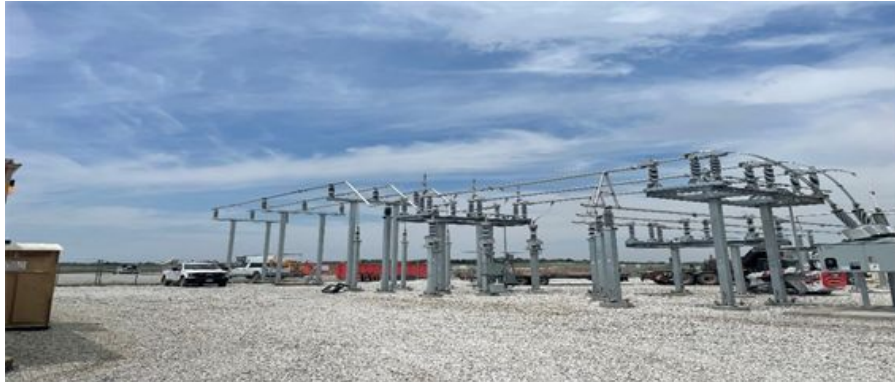
OPPD Substation – Bus Extension to AES Collector Substation
