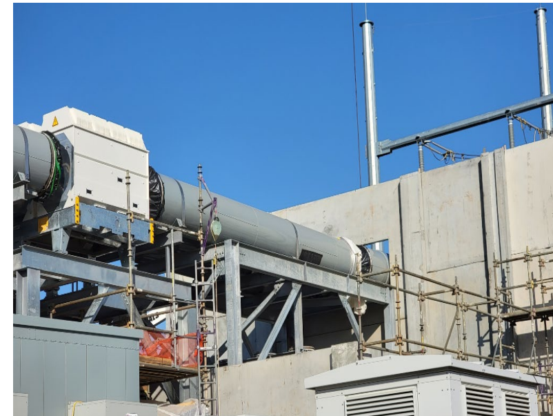
Facing Northwest – Unit #1 GCB/Isophase
