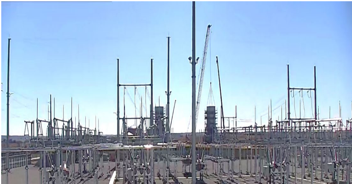
Facing South – Substation
