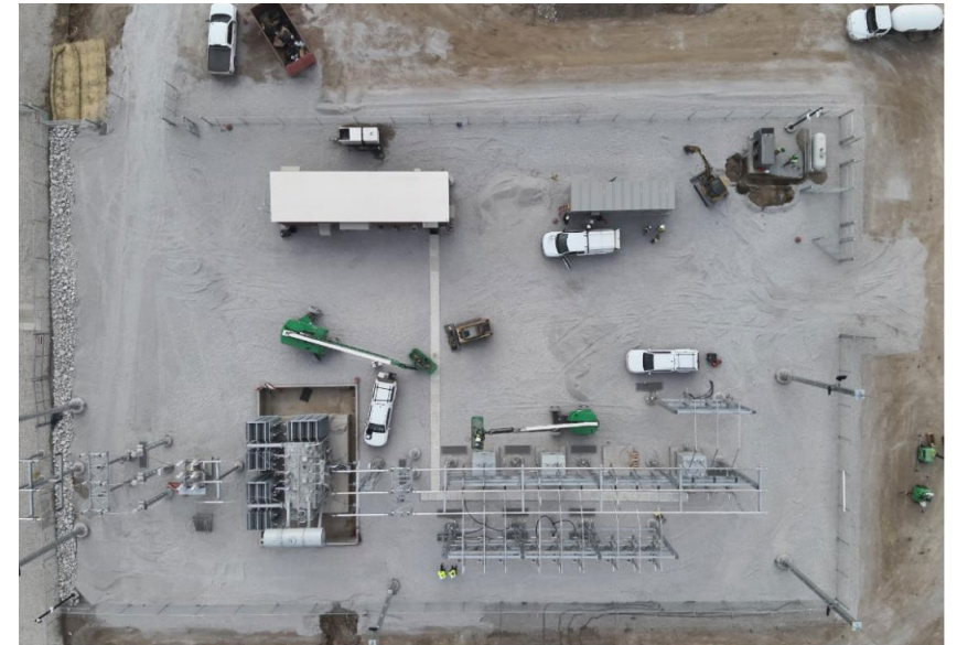
AES Collector Substation Operation
