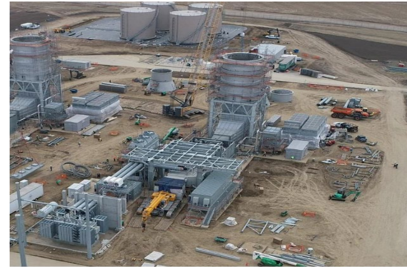
Facing South – Unit #2 Filter House Assembly
