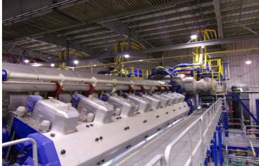
Facing East in Engine Hall – Top of Engine #9
