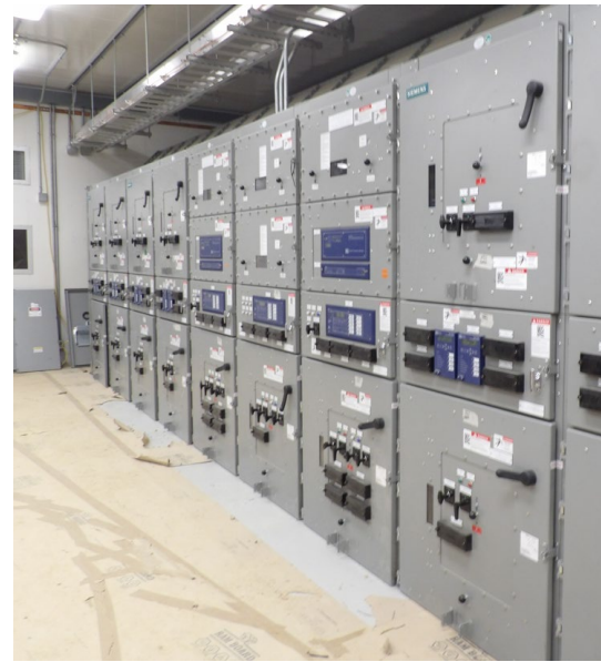
Power Distribution Center Motor Control Center
