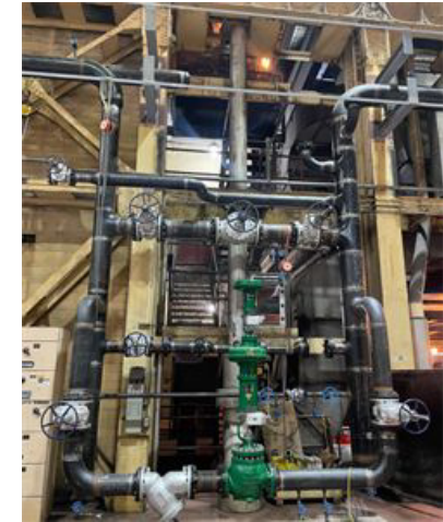
Auxiliary Boiler Piping
