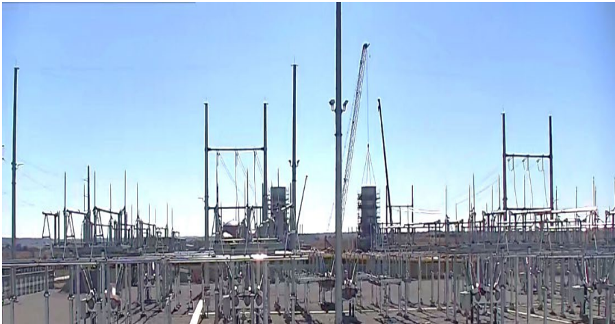
Facing South – Substation
