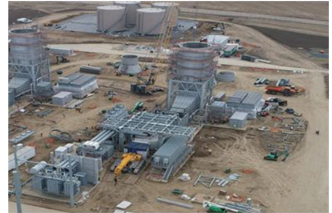
Facing South – Unit #2 Filter House Assembly
