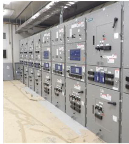
Power Distribution Center Motor Control Center
