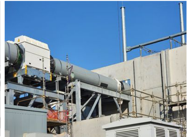
Facing Northwest – Unit #1 GCB/Isophase
