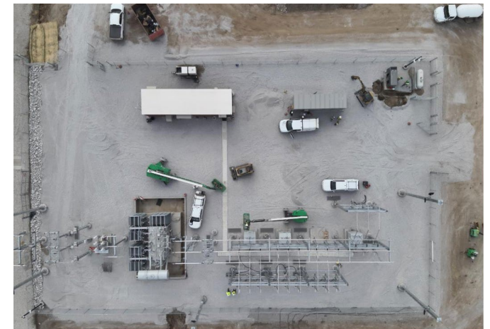
AES Collector Substation Operation
