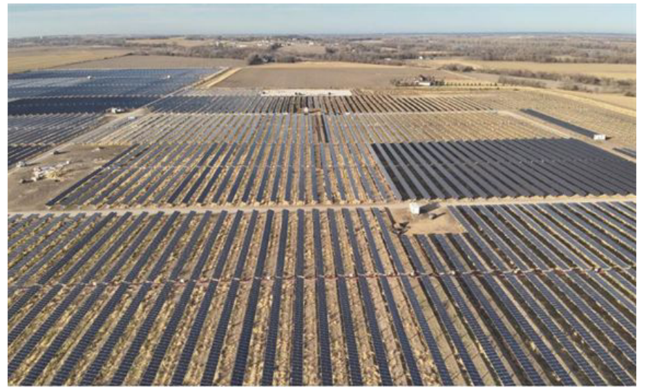
Platteview Solar – Aerial of South Parcel Nov 2023
